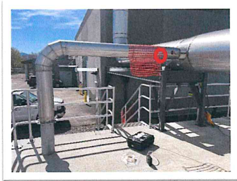
Aerobic Digester Exhaust
