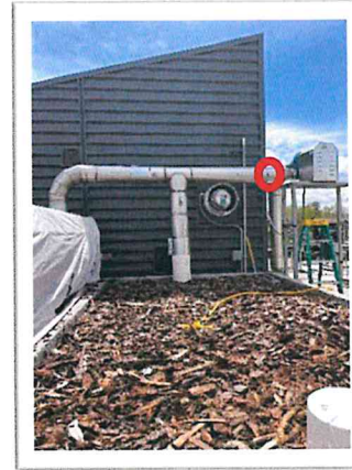
IPS Biofilter Inlet Duct
