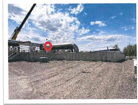
Biofilter Inlet Duct
